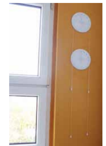
Natural ventilation unit in the reference room
