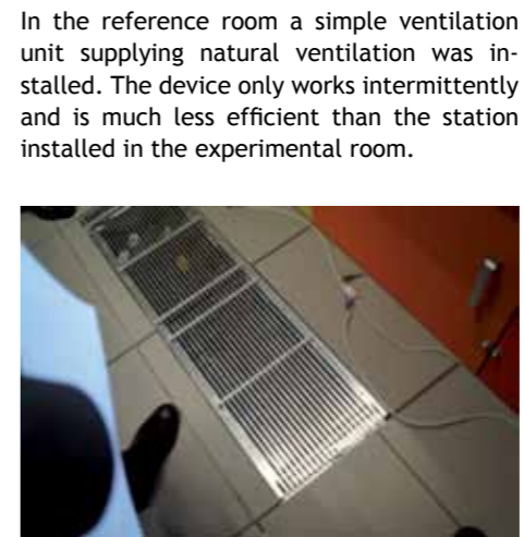
Underfloor ventilation station by TROX in the experimental room
