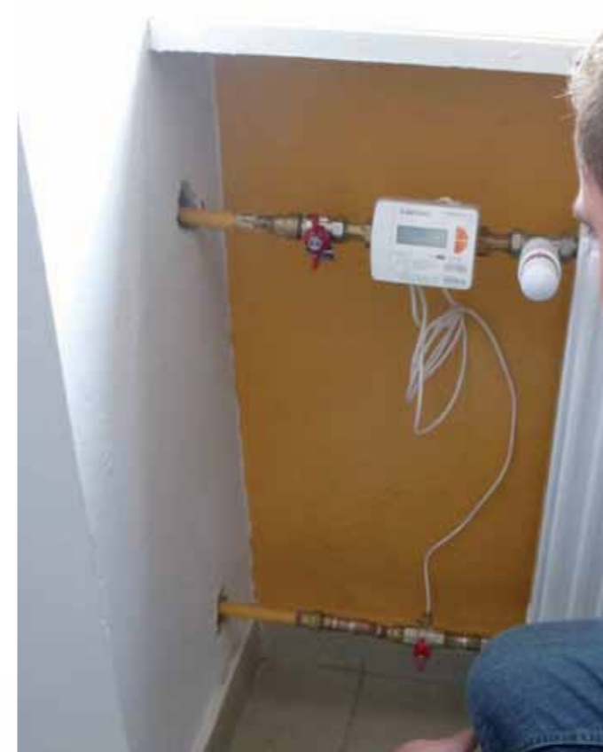
Measuring device for heating system
